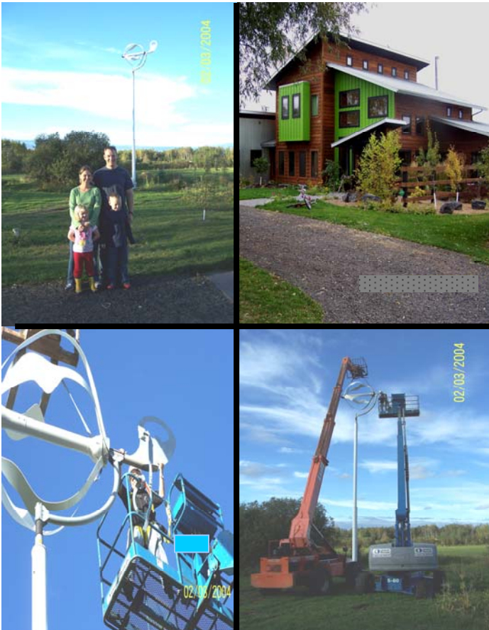
A V200 is installed at a rural residence in South Range, Wisconsin. Beautiful scenery, great weather, and happy customers; makes for a pretty good day.
