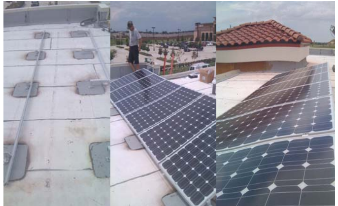
Another HEA Solar PV system is installed in Houston, TX by Gulf Coast Renewable Resources. Package design by Jon Trice, Installation executed by Justin Owens and the GCRR team.
